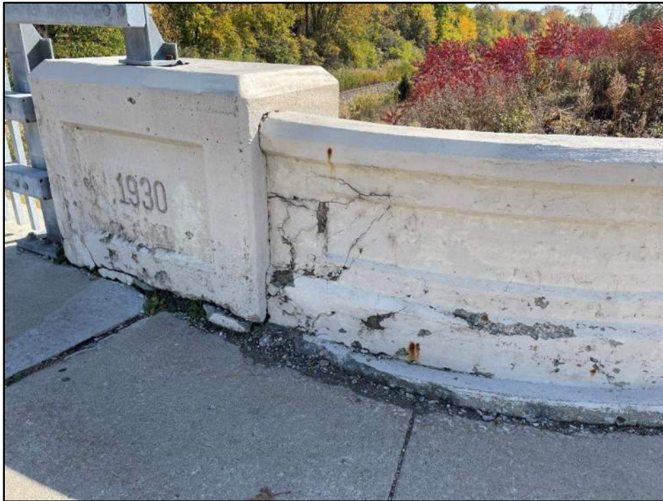
Sidewalk and spalls in concrete railing in southwest quadrant
