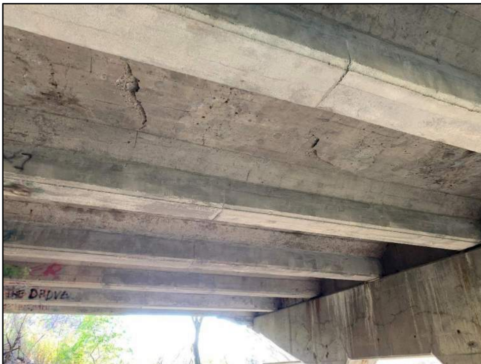
Deck delamination in east span
