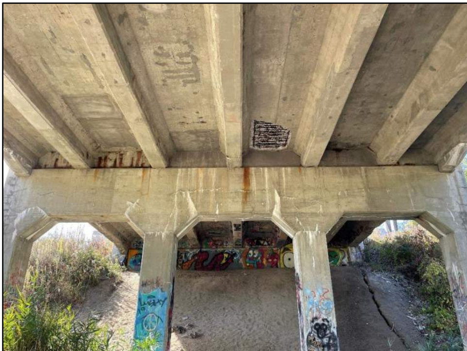
Deck spalls with exposed rebar and pier cracks in west center span
