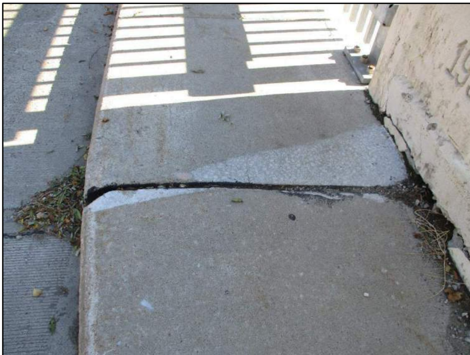
Sidewalk deterioration at abutment
