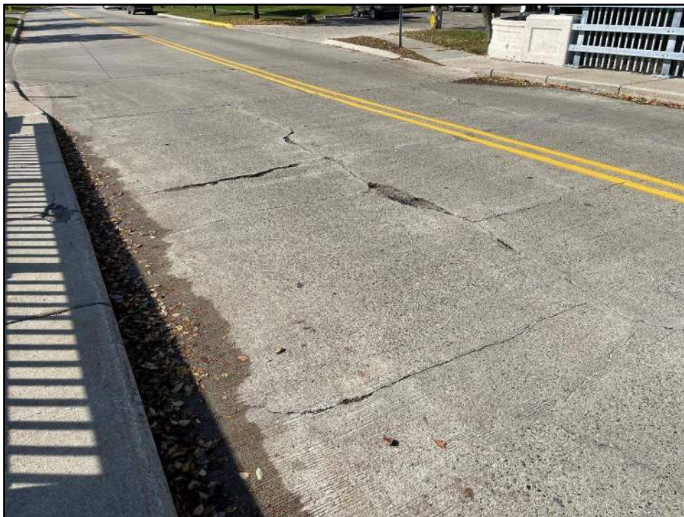
Longitudinal and transverse cracking in west span of bridge deck
