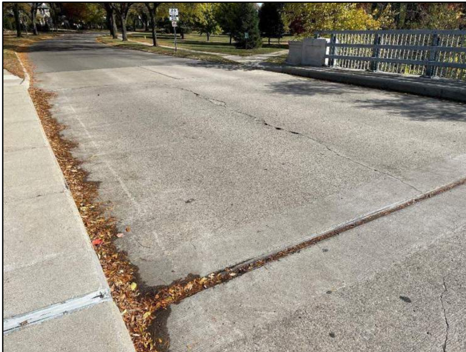
Longitudinal cracks and spalls in east span of bridge deck
