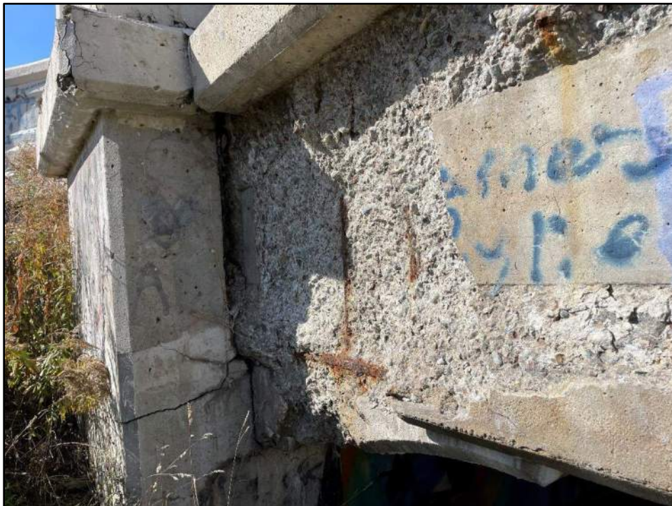
Spalls in fascia beam and abutment in southwest quadrant
