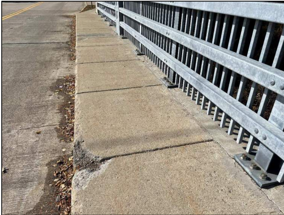
Spalling of north sidewalk
