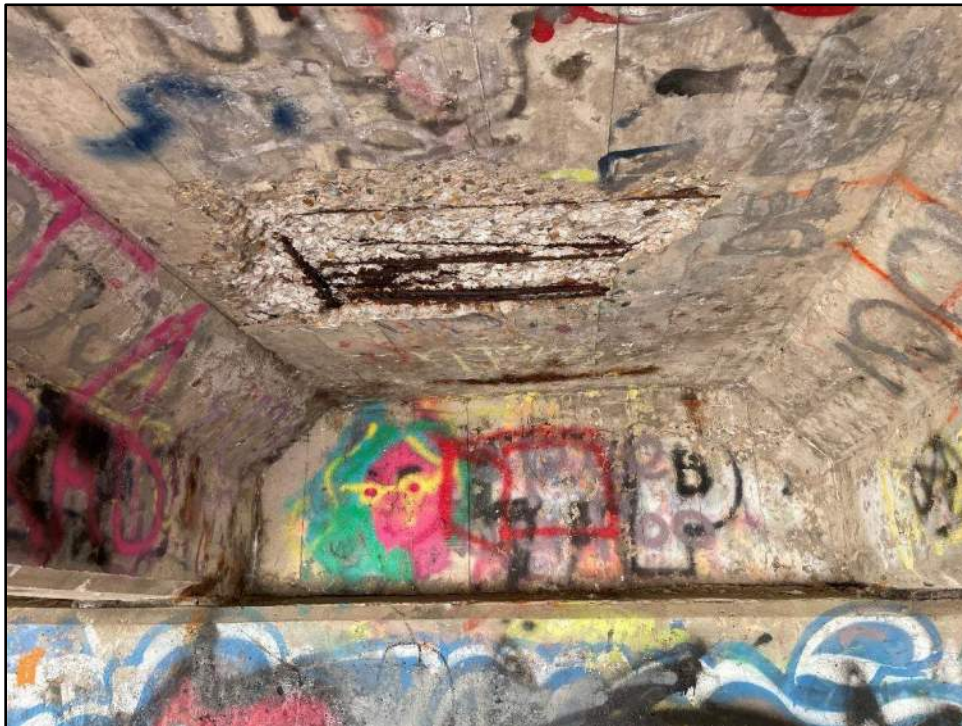
Deck spalls with exposed rebar in west span
