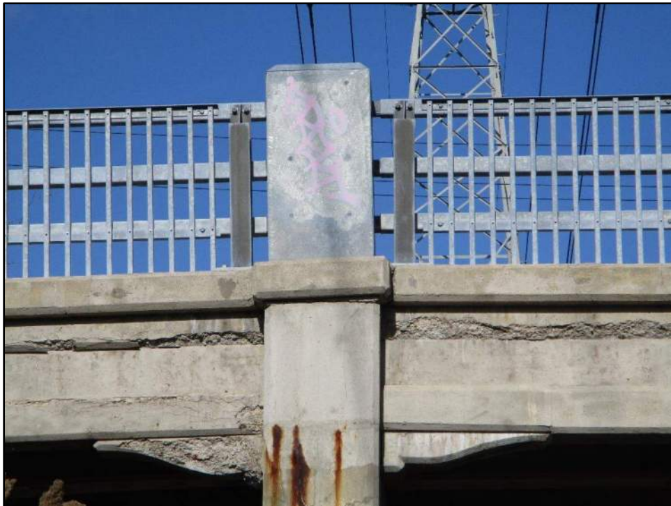
Deterioration on south fascia with out of plumb steel railing post at west pier
