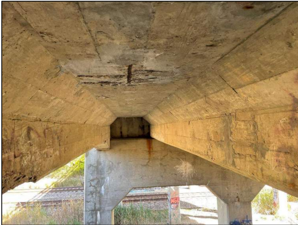
Deck spalls with exposed rebar, beam cracks and diaphragm deterioration in west span
