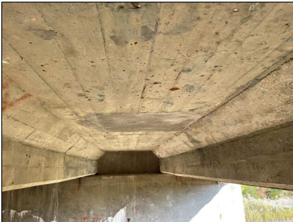
Cracking and delamination of previous repair in west span
