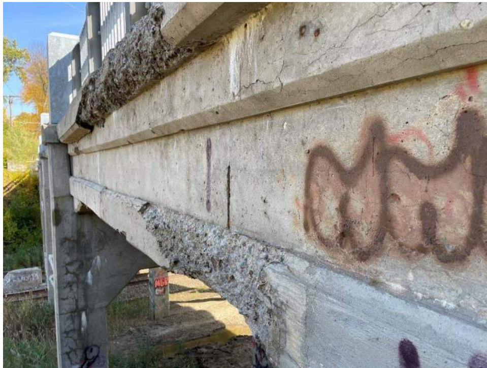
Spalls in sidewalk fascia and beam in northwest quadrant
